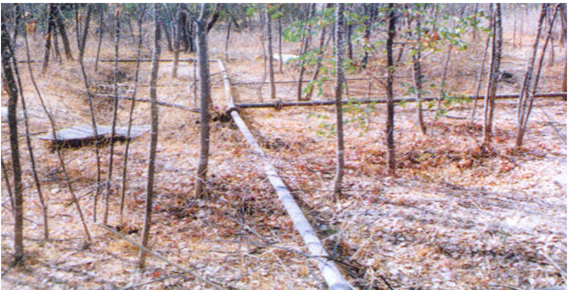
Pipeline for distributing collected water
